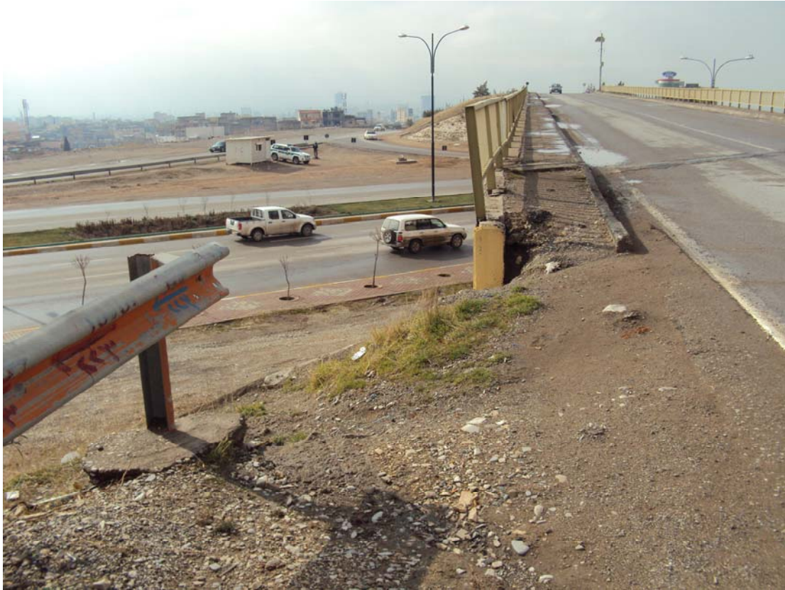
A gap between crash barriers
