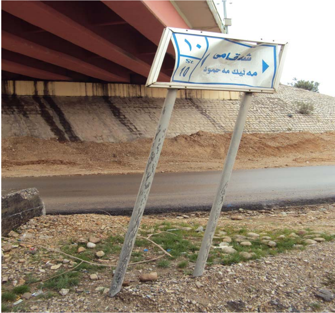
Road sign is also damaged which is considered as a part of the bridge ancillary.
