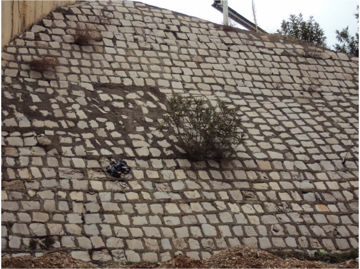
State of the wingwall, damaged rock face and plants are growing that could further damage the wingwall.
