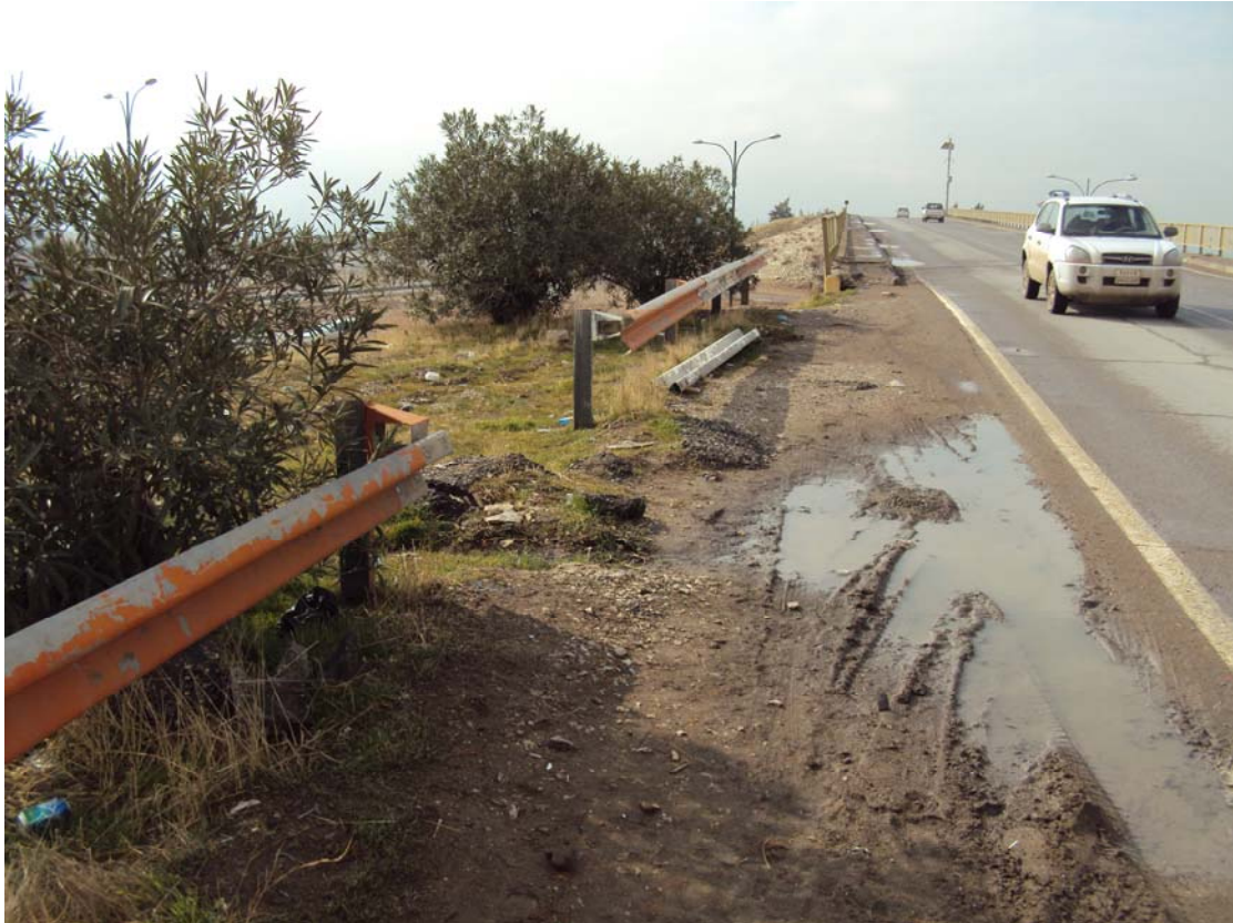
Crash barrier, sign of accidental damage but it was not repaired
