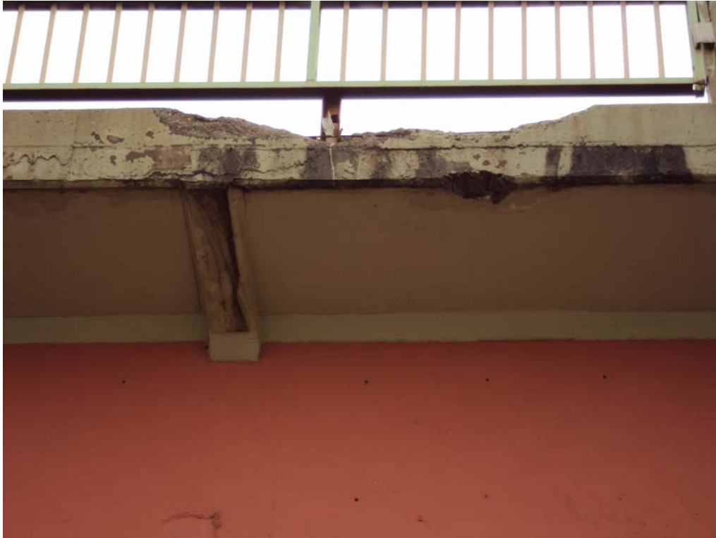
Crash barrier over the bridge, sign of accidental damage but it was not repaired properly and still poses a risk to the bridge users.
