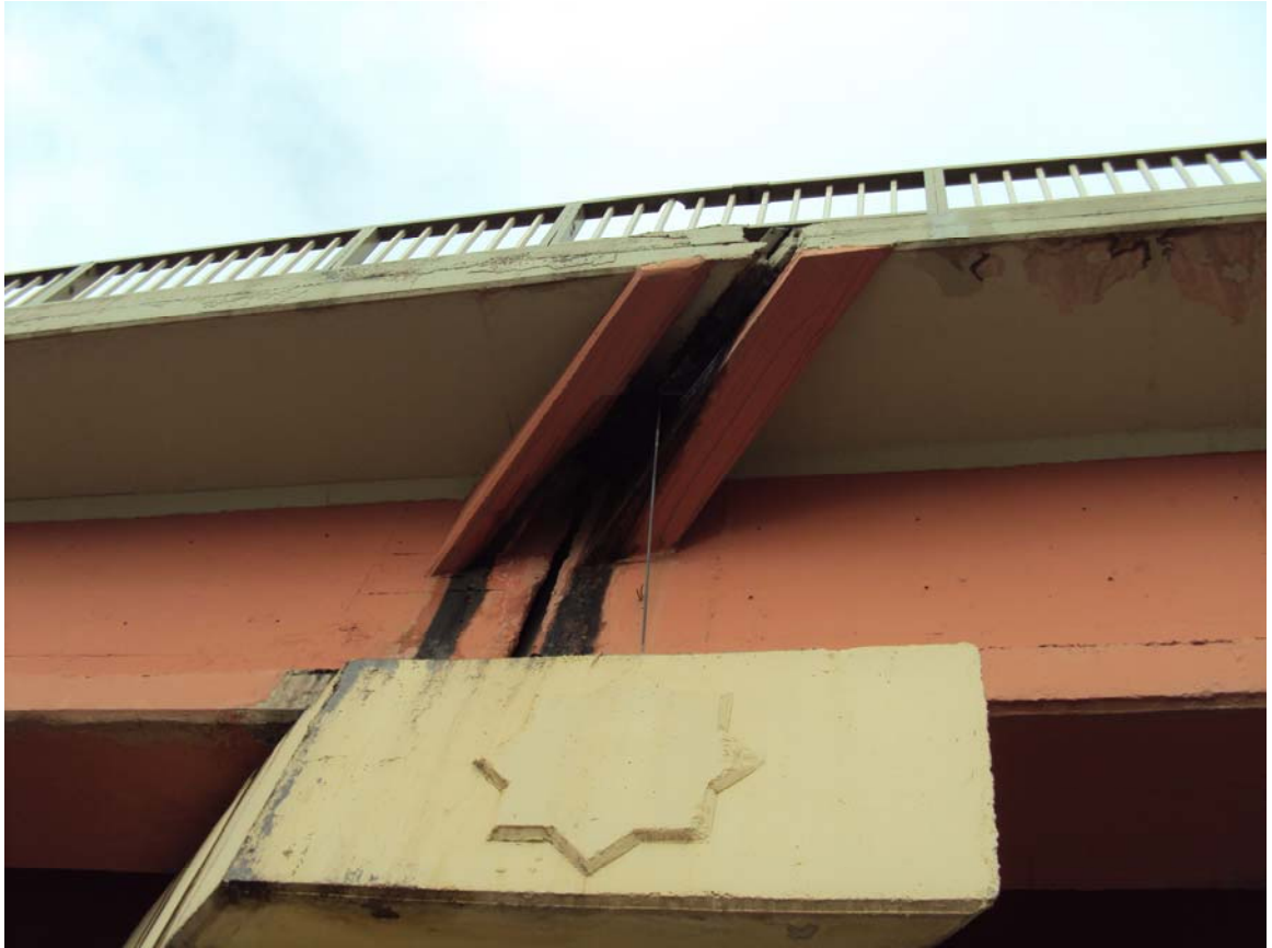
Expansion joint fill is deteriorated and needs to be replaced and sealed properly to prevent further damage.
