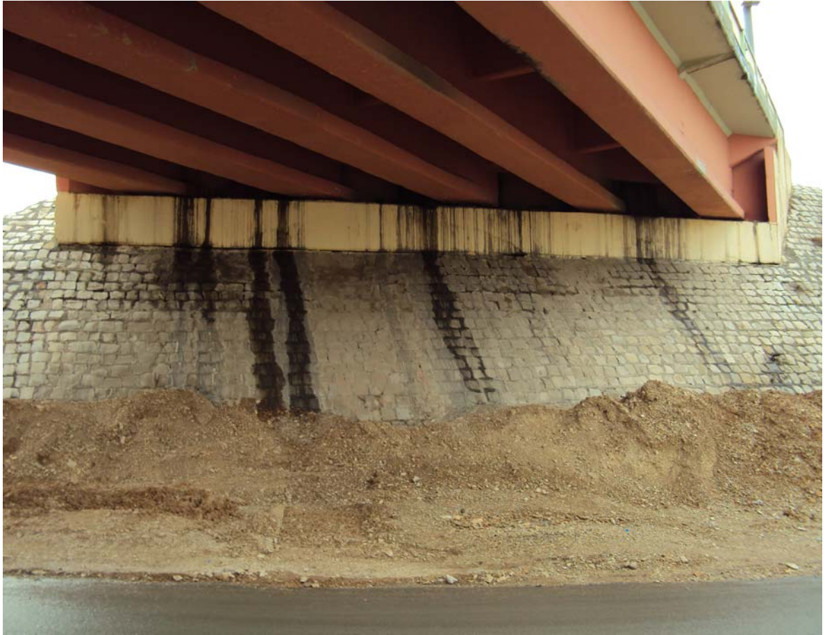
Rock face of the abutment, there are signs of spalling and cracks. Leakage can be seen running down the abutment. Damp proof memberance is required to stop the leakage.
